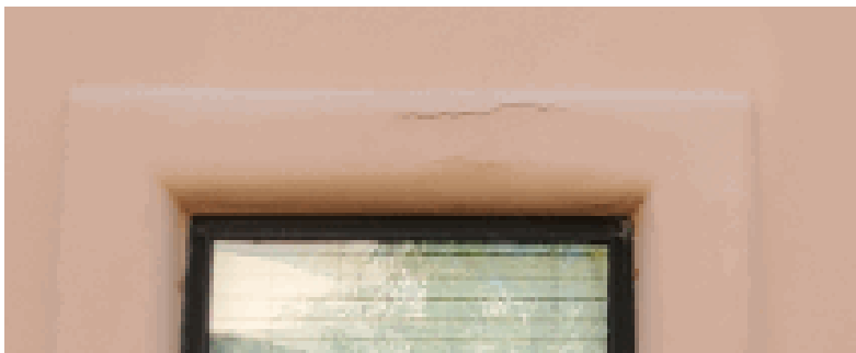
Cracks large enough for potential water incursion-west side
