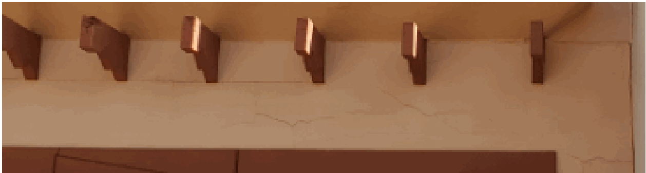
Crack after 10-year-old repair-south side
