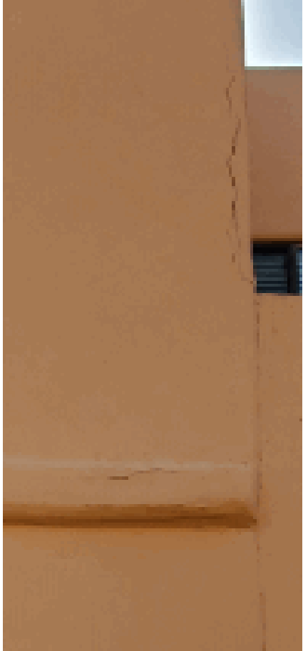
Cracks in several directions-west side
