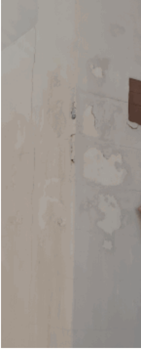
paint peeling-west side
